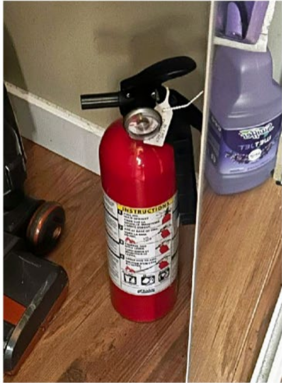
Fire extinguisher is in the hall closet.
